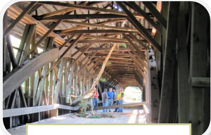
The branch went through the roof as well.
