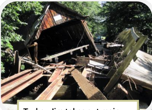
Turkey Jim takes out main bridge to Branch Brook
